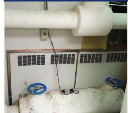
FIGURE 1 Dead leg (bottom) located in a closet in a basement.
