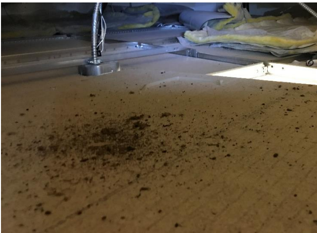
Photograph 1: Debris on top of ceiling tiles.
